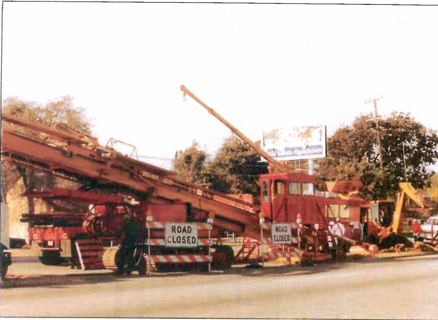
Davis' crew conducted the directional bore successfully for Oklahoma Natural Gas and achieved their goals of causing a minimum of disruptions to this busy area of Tulsa.
