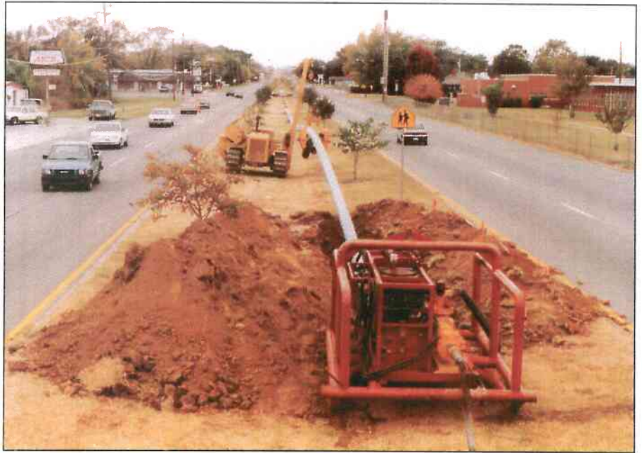
Davis Corporation of Healdton, OK, recently completed a difficult directional drilling job in Tulsa, OK. Among the obstacles to overcome was having to locate their bore pits in a narrow center median of a busy street.
