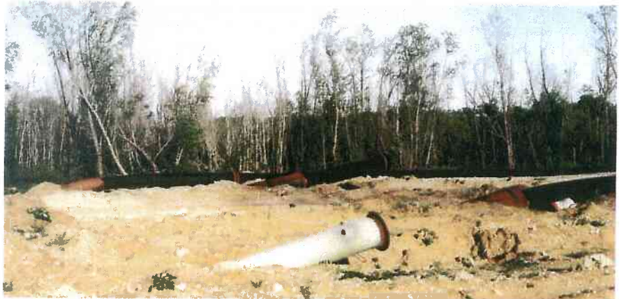
Three completed 20-inch conduits and one 10-inch conduit were involved. The 20-inch conduits contain 16-inch polyethylene pipe. The 10-inch conduit will have communication cable installed.
